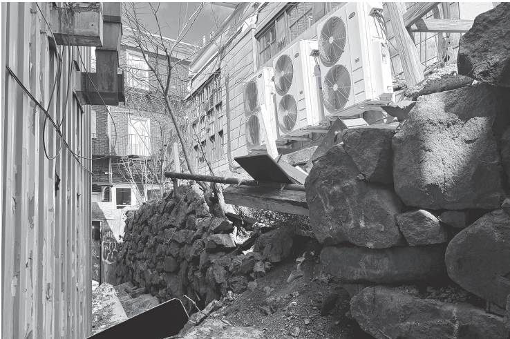
The collapsed segment of a historic wall in the Harvard Square alleyway between the former Red House and the IHOP, parallel to Eliot Street.
